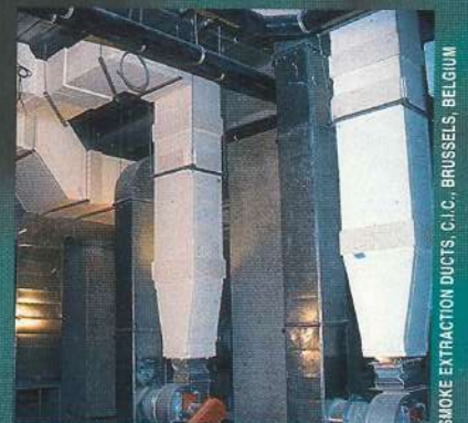
SMOKE EXTRACTION DUCTS, C.I.C., BRUSSELS, BELGIUM
